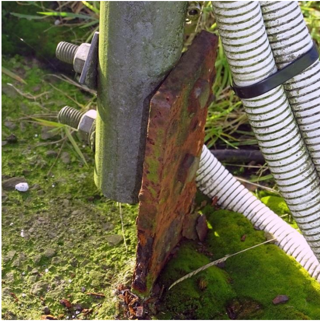
Rusted N/E tower footing, photographed May 2024
